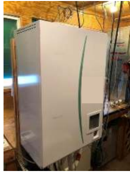
DX to water HXer, pump, controls
