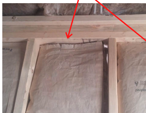
Significant gaps and insulation does not fill entire cavity
