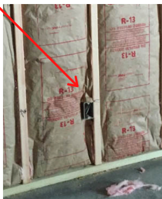
Insulation is not cut around electrical box
