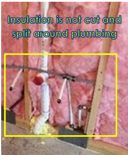
Grade III: Not Compliant
