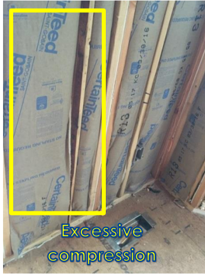
Grade II: Not Compliant
