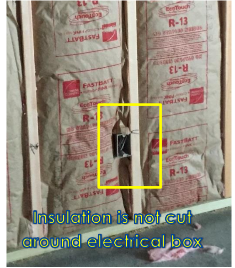
Grade II: Not Compliant
