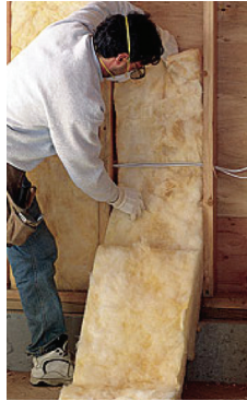
Insulation is cut and split around electrical wiring
