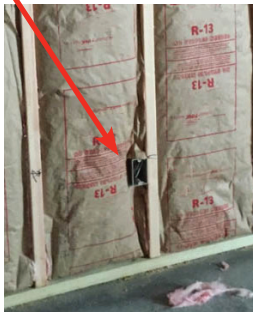
Insulation is not cut around electrical box
