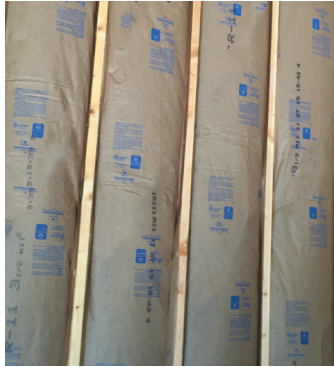
No noticeable gaps or compression
