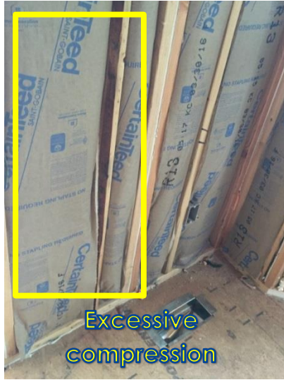
Grade II: Not Compliant
